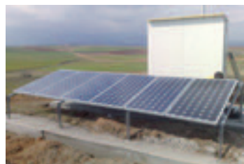
Solar Photovoltaik Telekommunikationssystem Solar photovoltaic telecom system
