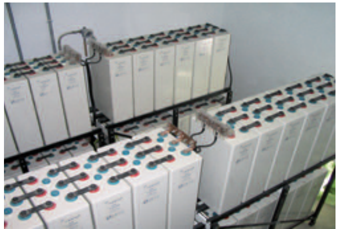
Solar photovoltaic industrial system
